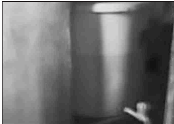
The Water purifier (converting air into water) was installed at DMS Alamadhi Centre. The Donor is Akash Ganga AME india Pvt Ltd. The cost is Rs.38,000
